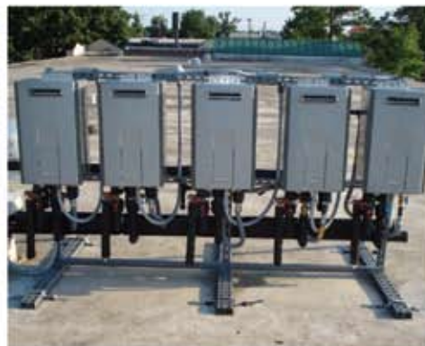
At this 40-room hotel, exterior units are mounted on the rooftop with no additional venting. Hotel owners have experienced 50 percent reduction in therms per occupied room.
